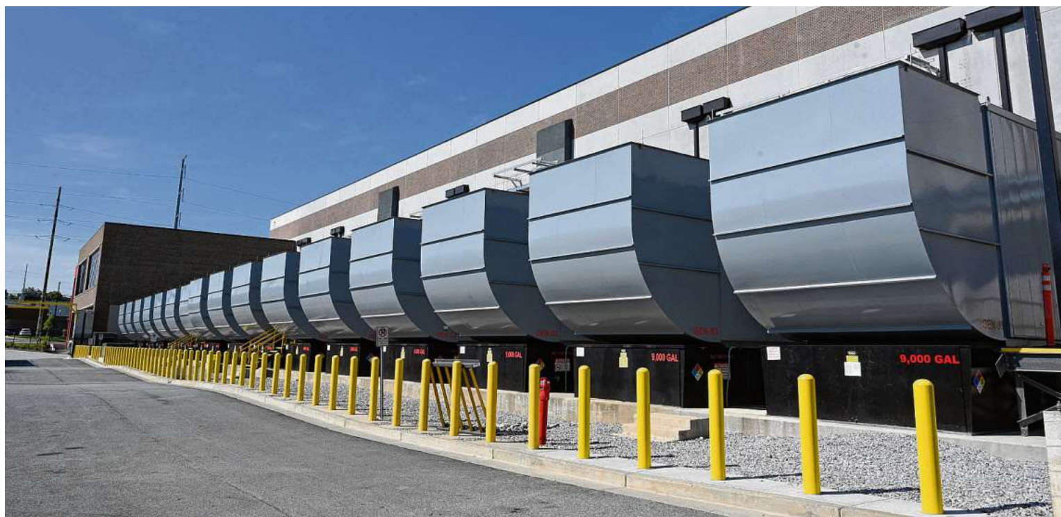
The QTS Atlanta Data Center has its own Georgia Power substations. Georgia Power has outlined plans to meet a 50% jump in power demand by 2035, driven largely by rapid expansion of data centers, expected to account for over 80% of new large-customer power demand. HYOSUB SHIN/AJC 2022
